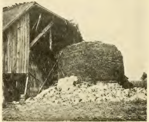
This Vitrified Tile Silo Collapsed First Night After Filling. On Farm of Neff Wildrick, Colusa, Ill.
